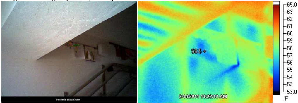
Image 3b: Emergency stairs, inadequate insulation
