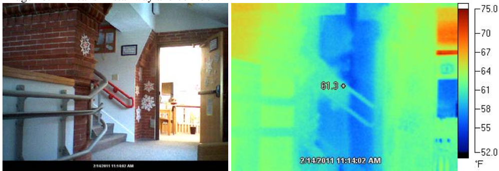
Image 4b: Air leaks in stairway and corridor
